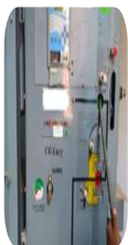
Servicing, Testing and Periodical Inspection of 11kV Electrical substation with 350KVA Oil Cooled Transformer and CG Lucy VCB
