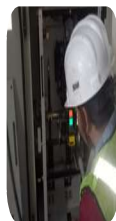
Testing and Periodical Inspection of 11kV Electrical substation with 750KVA, Oil Cooled Transformer.
