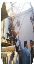
Servicing, Testing and Periodical Inspection of 11kV Electrical substation with 630 KVA (DELHI NCR)
