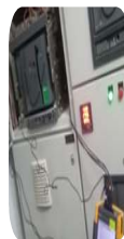
Servicing, Testing and Periodical Inspection of 11kV Electrical substation with 400KVA Oil Cooled Transformer with Ashida Relay
