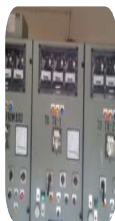
Testing and Periodical Inspection of 11kV Electrical substation with 1000KVA, 2 Dry type Transformer and Siemens relay
