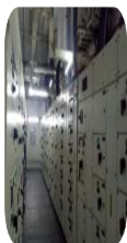
Servicing, Testing and Periodical Inspection of 11kV Electrical substation with 630KVA Oil Cooled Transformer with Merlin Gerin relay
