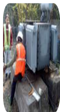
Testing and Servicing of 160KVA Transformer with OLTC, 11kV Isolator Panel, HT & LT Cables (DELHI NCR)
